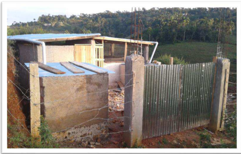
Image 4. A view of the pig pen and courtyard after laying of multiple block layers.
