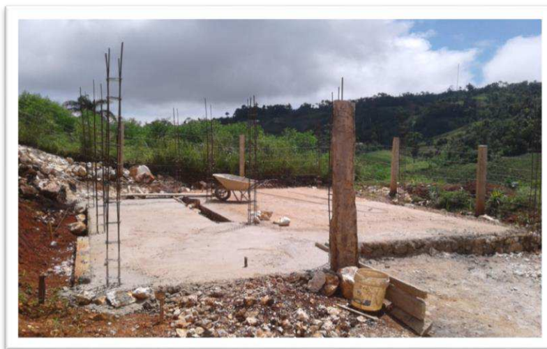
Image 1. View of the foundation and support posts taken early during Phase 2 activities.
